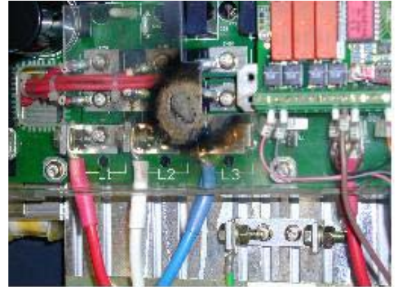
Damage caused by condensation
